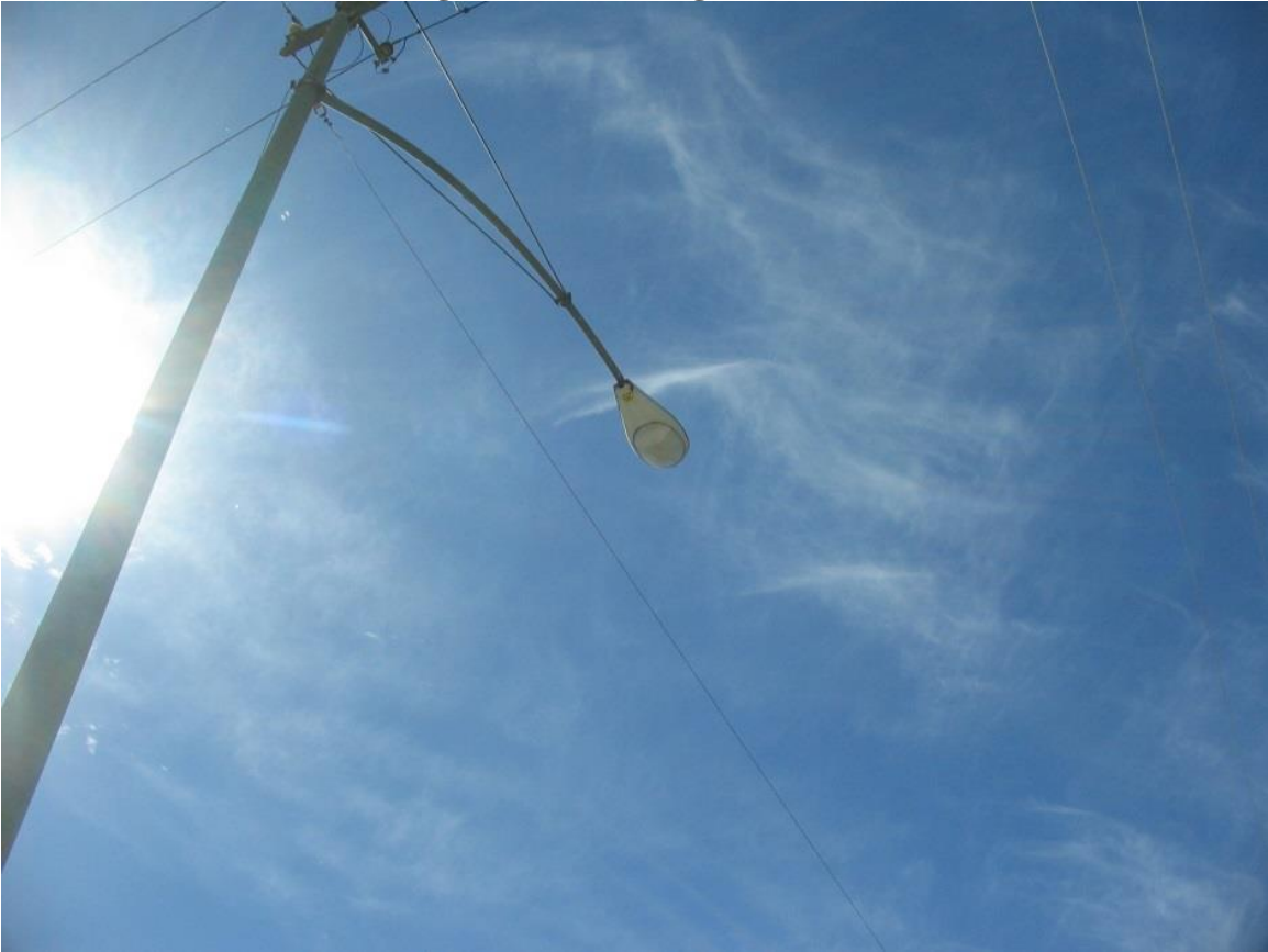
Existing streetlight located on Highway 111
